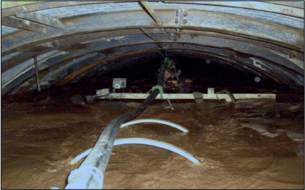
Photo: Parbati TBM buried in silt
